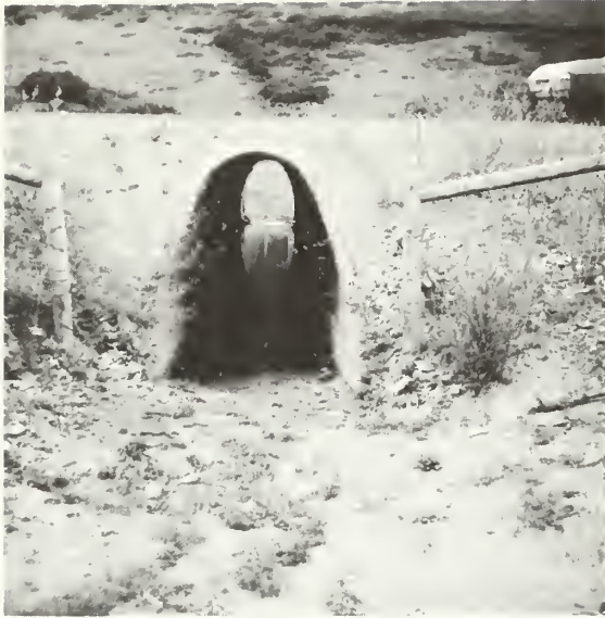
EAST ENTRANCE; 6" of water
